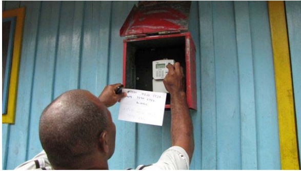
Prepaid electricity supply system
