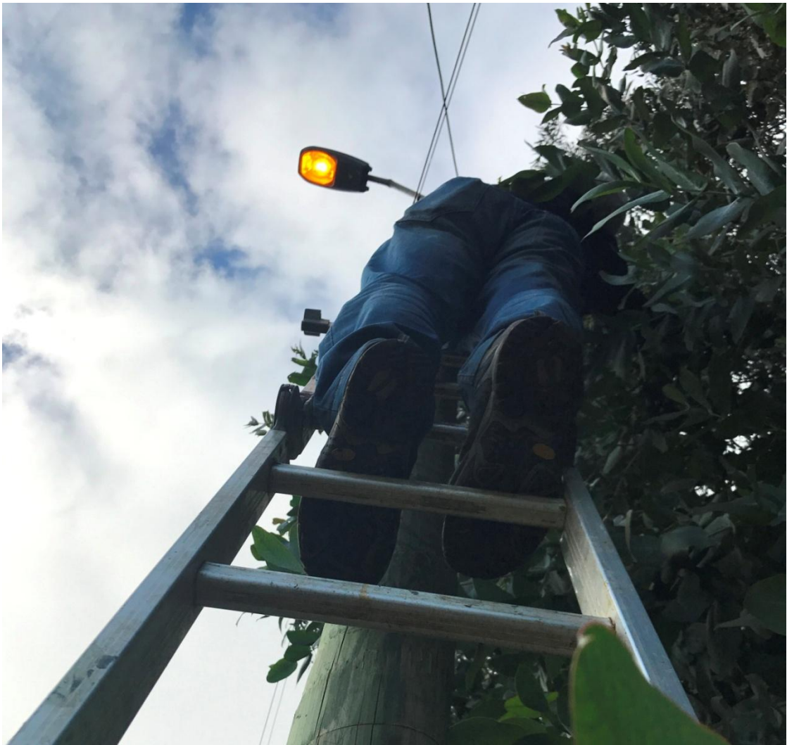
We are checking the lamps outside of the bungalow
