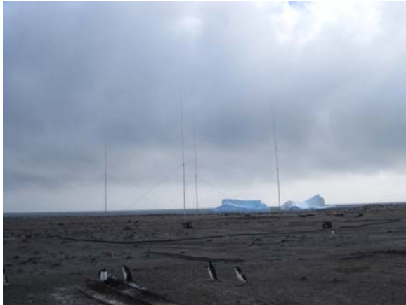
Our 40 meter four-square array with passing ice bergs in the background.
