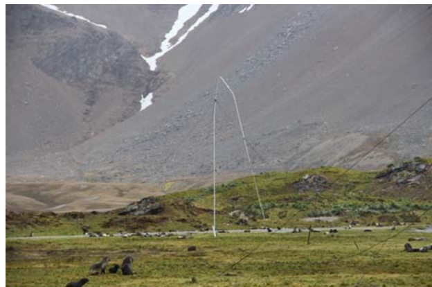
One of our phased 160 meter vertical antennas destroyed by high winds.
