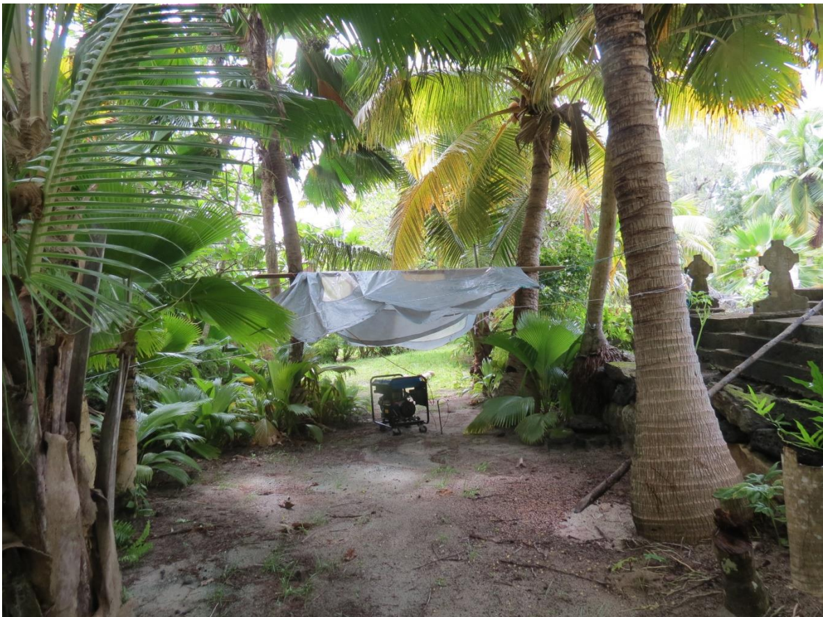
The 3KVA Diesel generator located some distance away from the shack, to lessen the impact of the noise. Note the tarpaulin to keep the rain away, and the proximity of the village graveyard.
